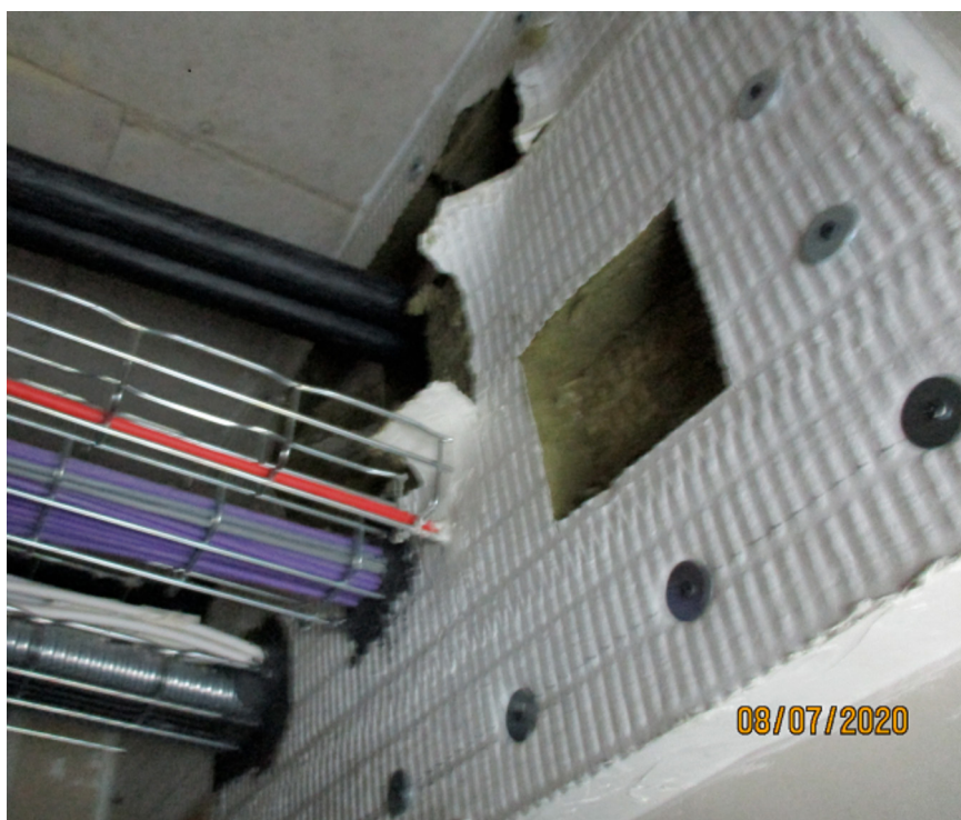
New services being fitted through existing seal – manufacturer unknown; original seal likely to provide appropriate period of fire resistance when remediated and appears to be correctly installed.
